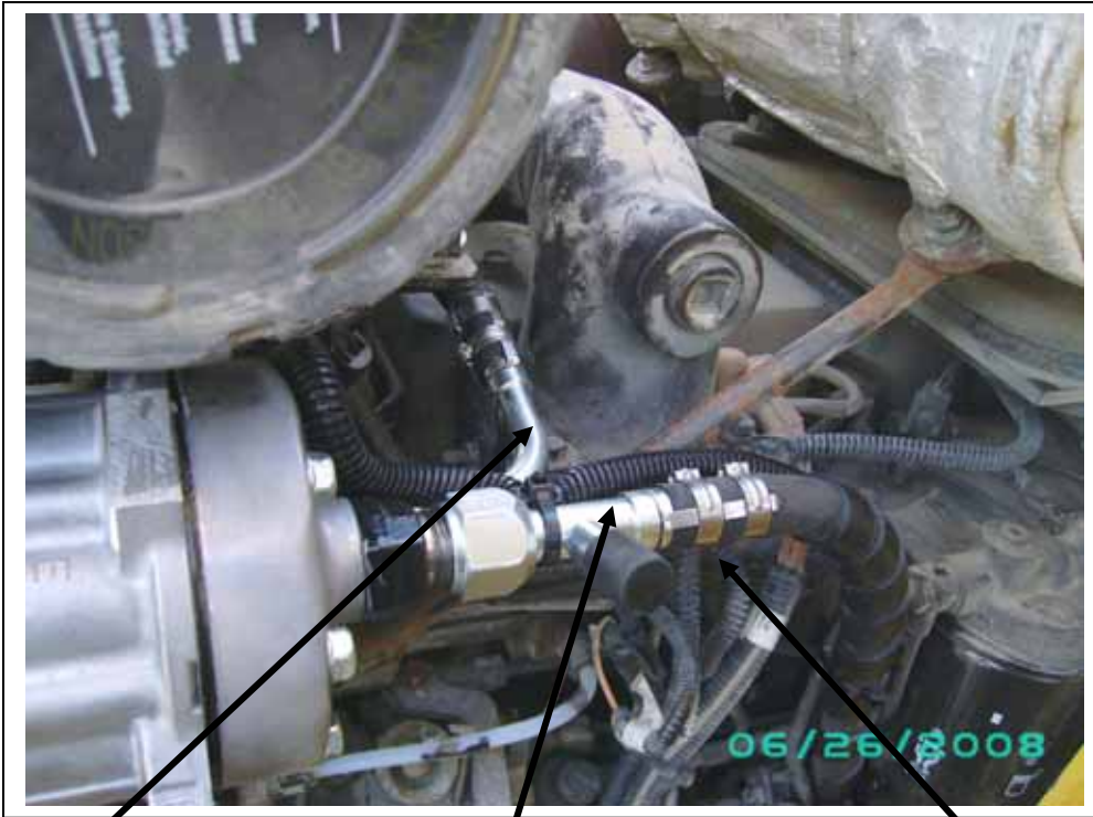
13/32" 90° female fitting on discharge side of compressor.
