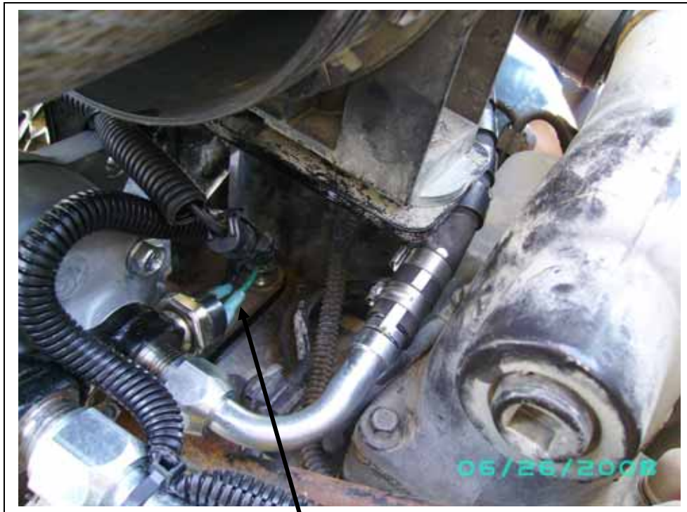
Clutch wire connected to the binary switch at the compressor.
