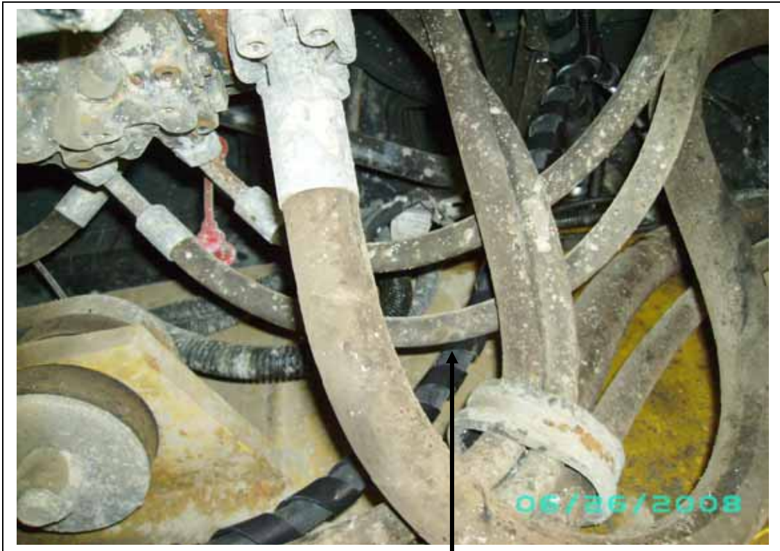
5/16" line heading up towards the evaporator under the cab.
