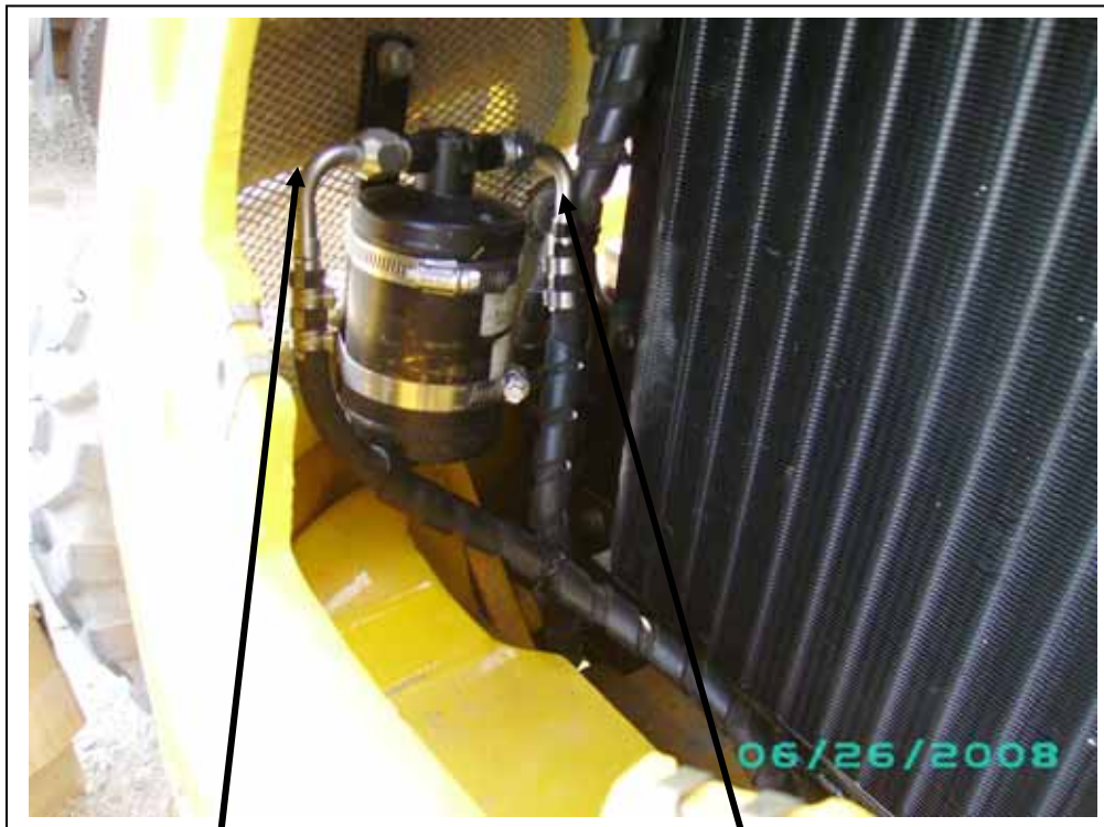
5/16" 90° female fitting at drier inlet from condenser.
